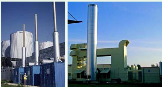
Pro2 power generation hardware at left and a new turbine at Claye-Souilly in Veolia ES photos
